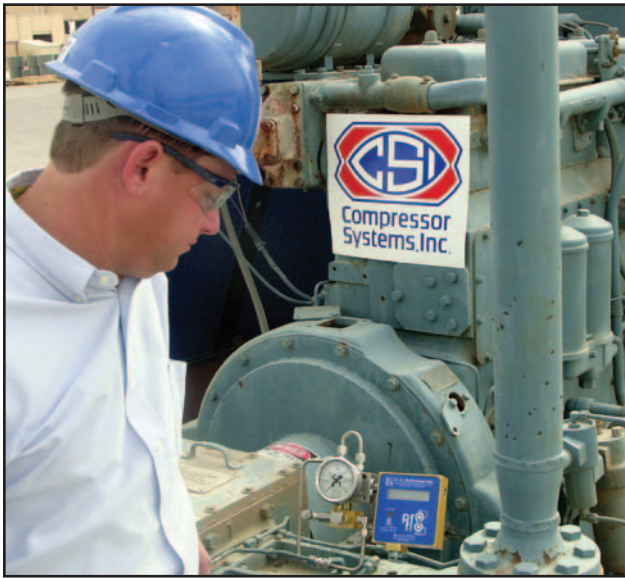
■ A Compressor Systems Inc. mechanic overlooks the operation of a Single Point Test Device on this Ariel compressor. CSI's Lloyd Roberts said monitoring oil is a way to manage maintenance costs.
